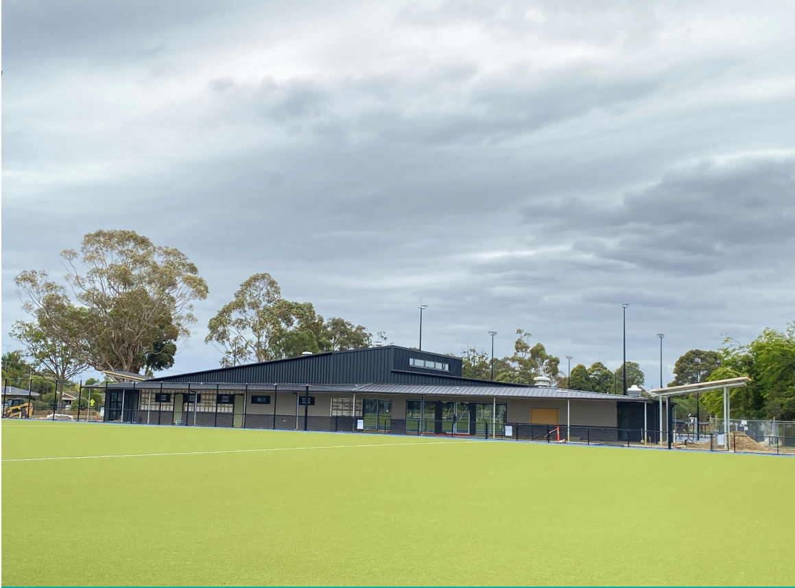
The pavilion at the WORLD Sporting Precinct, is taking shape, with an expected completion date pencilled for May 2024
