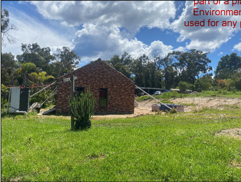
Image – New dwelling in construction and existing outbuilding to remain to Lot 1.
