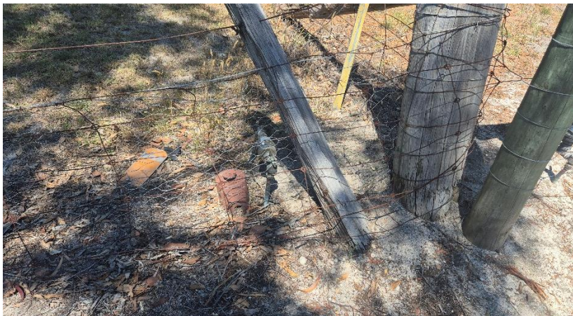
Existing water metre
