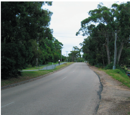
Stormwater flows directly along main road
